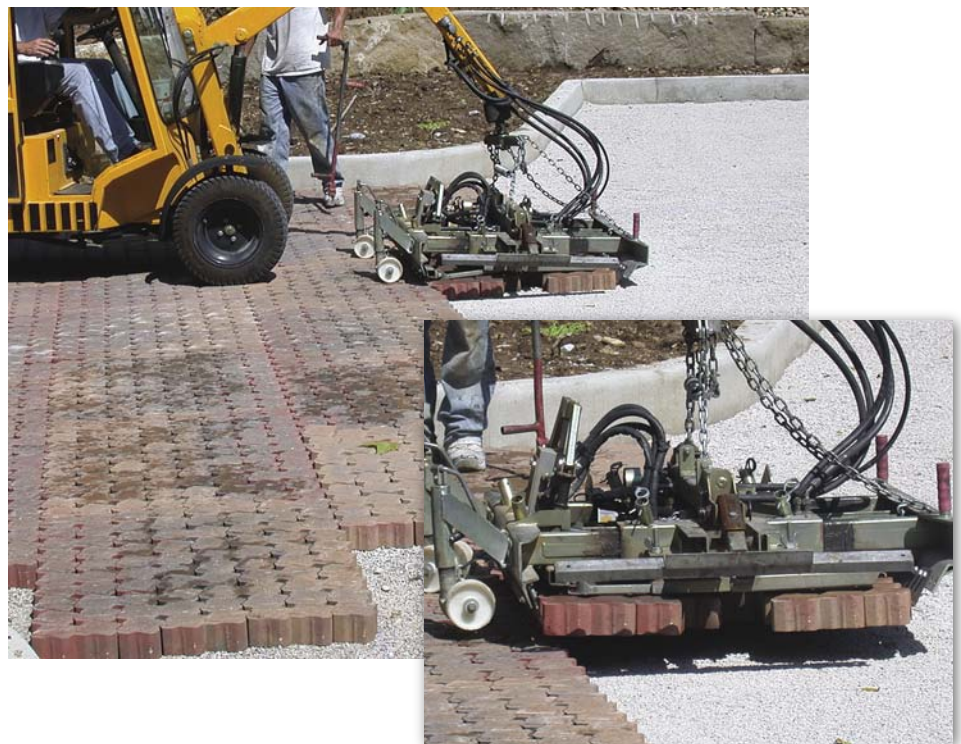
Figures 3 and 4. Permeable interlocking concrete pavement was mechanically placed over a 2 in. (50 mm) of chip gravel, a 4 in. (200 mm) thick base of No. 57 stone 5 in. (125 mm) thick No. 2 stone subbase.
