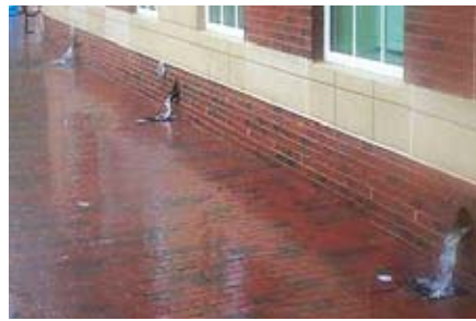
Rams Head Plaza at UNC Chapel Hill features an underground cistern. Above, downspouts convey roof runoff into the plaza inlets. The water is stored and later used to irrigate plaza plants. photo: http://sustainability.unc.edu
