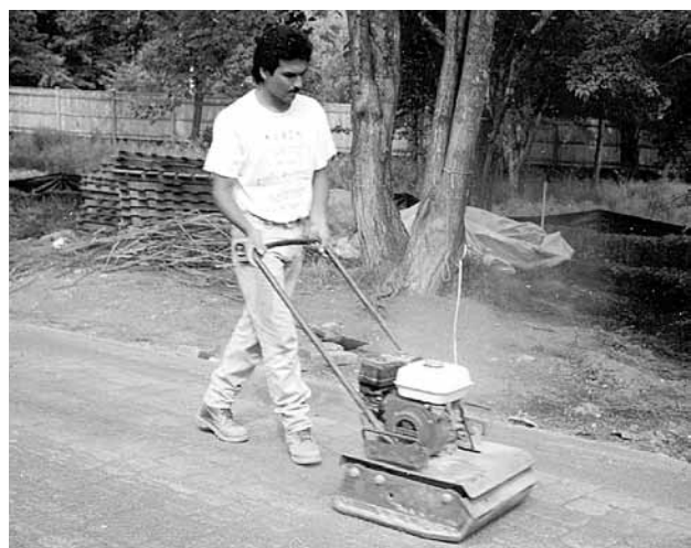
Figure 9. Final compaction of the pavers and settling of the sand into the joints.
