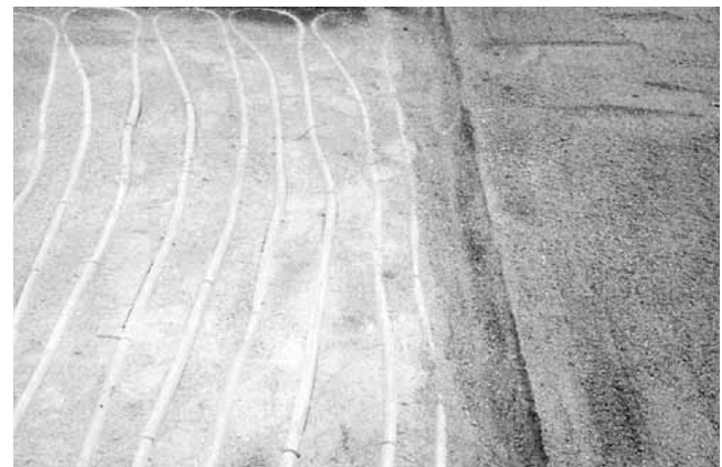
Figure 7. Screeding bedding sand must be done without moving or damaging pipes or wires for melting snow.
