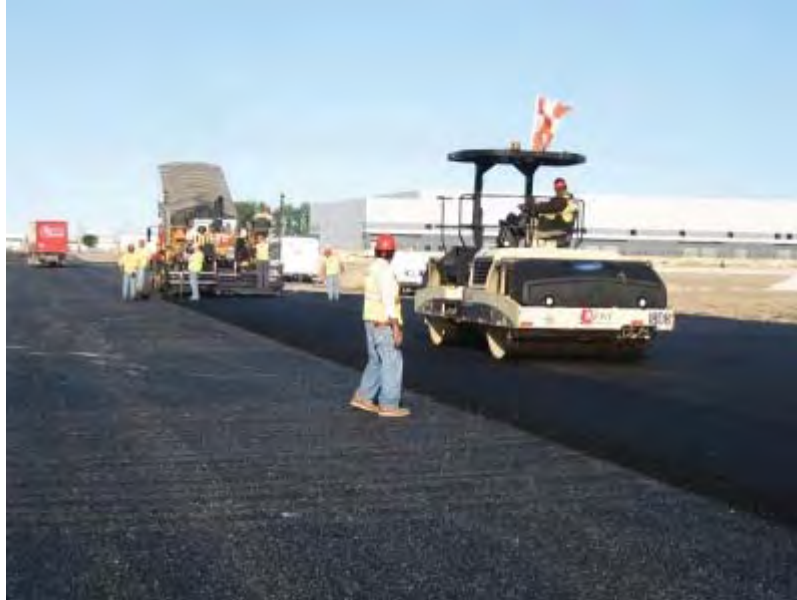
Figure MR-1.2: June 2010 Runway 10C-28C Paving and Electrical (West): Placing and compacting Bit concrete base course on taxiway (Photo Courtesy Chicago O’Hare Modernization Program)
