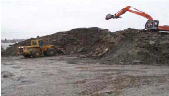
Figure PR-6.2: Typical pile of roadway construction waste. (Bremner & City of Vancouver, 2006)
