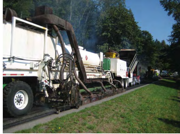
Figure MR-2.14: HIR equipment heating and removing the top layer of existing HMA.
