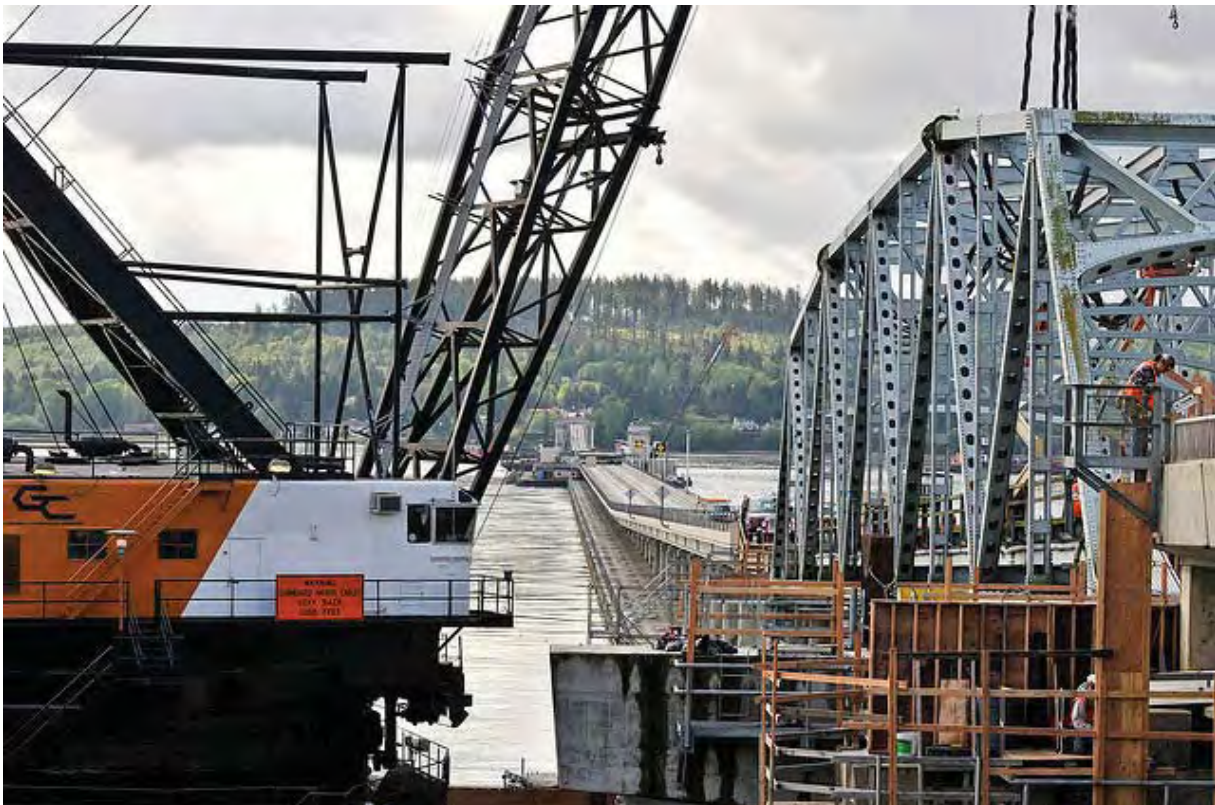
Figure MR-2.6: Hood Canal floating bridge retrofit and replacement project. (Photo Courtesy of WSDOT)
