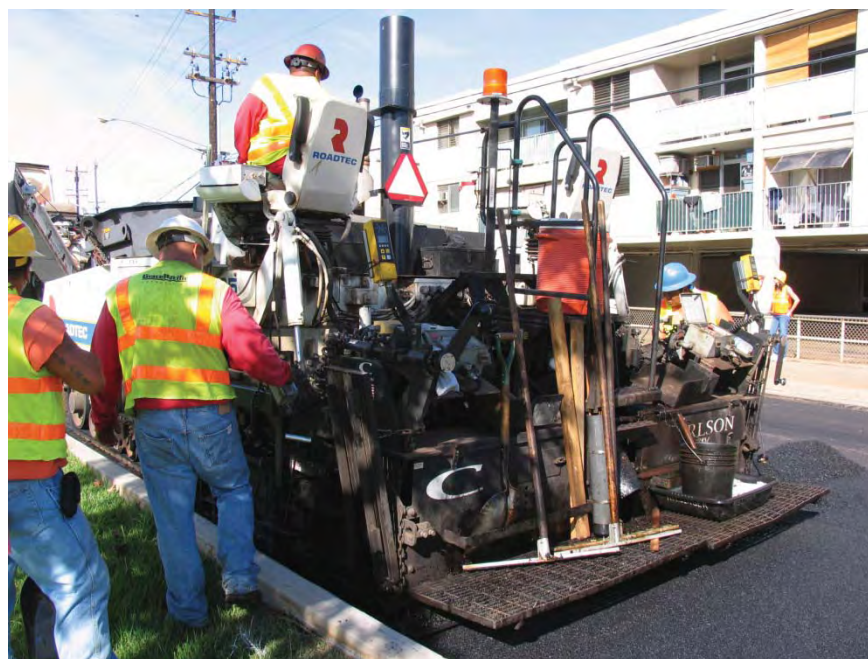
Figure CA-6.2: The large black exhaust stack to the right of the operator is part of a NIOSH compliant exhaust ventilation system.
