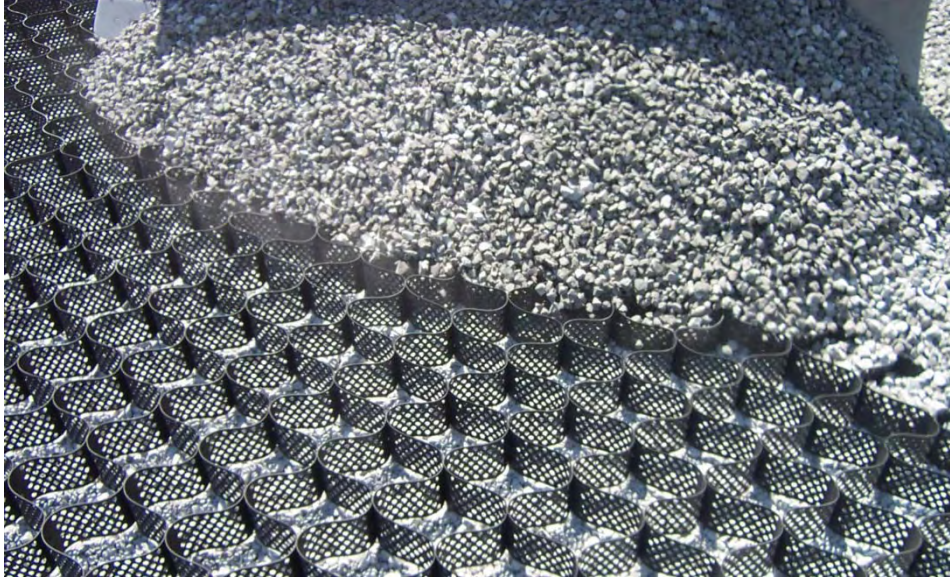
Figure PT-2.7: Turf reinforcing grid installed in gravel parking area in Pennsylvania to alleviate ponding issues. (Blair County Conservation District, n.d.)
