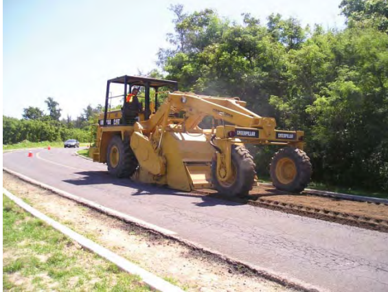
Figure MR-2.16: Road reclaimer used in FDR (photo from Grace Pacific, Inc.).
