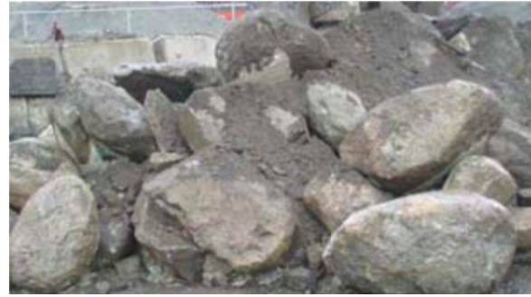
Figure PR-6.3: Boulders excavated during roadway utility work. (Bremner & City of Vancouver, 2006)
