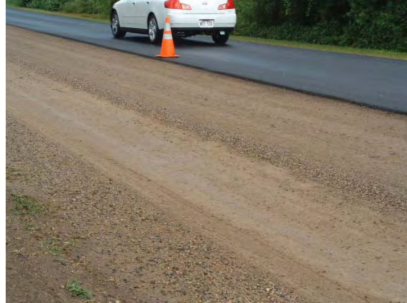
Figure MR-2.17: Finished FDR material before overlay (photo from Grace Pacific, Inc.).
