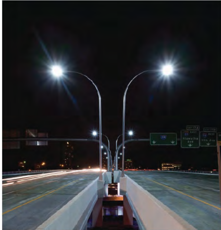
Figure MR-6.2: Lit LED luminaires at night on I-35. Photo by Figg Engineering Group. http://www.ledwaystreetlights.com/Benefits/pdf/case-study/ledway-I-35W-CaseStudy.pdf
