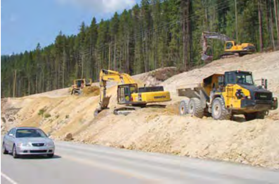
Figure MR-3.4: Phase 3 of The Kicking Horse Project: Excavation on north side of the highway (BCMOT, 2010)
