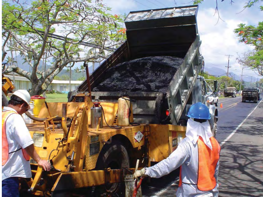
Figure CA-6.3: This paver is NOT equipped with an exhaust ventilation system.
