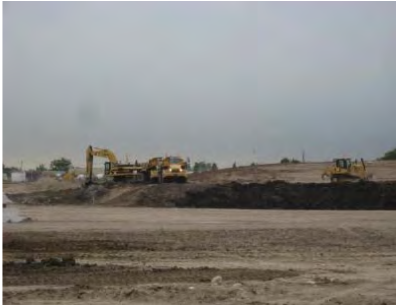
Figure MR-3.1: Runway 10C-28C Paving and Electrical (West): Excavation in Area G5 (Photo Courtesy Chicago O'Hare Modernization Program)
