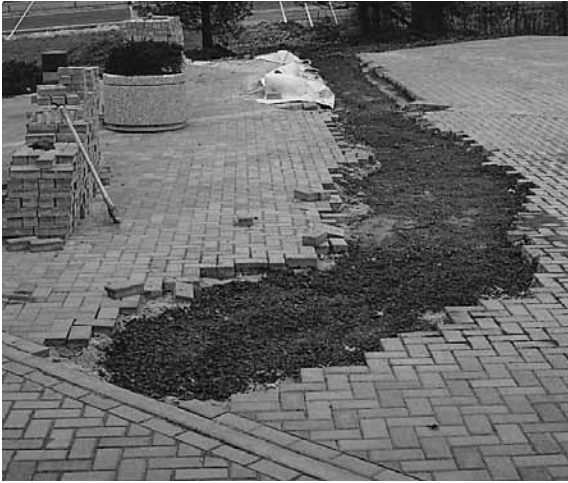
Figure 11. Trench filled with compacted aggregate base. Temporary edge restraints should be used around the opening perimeter.
