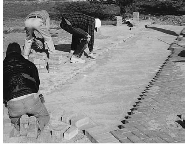
Figure 12. Screeded bedding sand. Note that a few courses of pavers are removed to create even sides for screeding. Installing temporary edge restraints prior to excavating is preferred practice.
